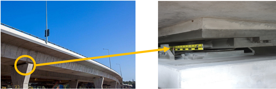
Figure 2. Seismic isolation bearing at Newmarket Viaduct.
